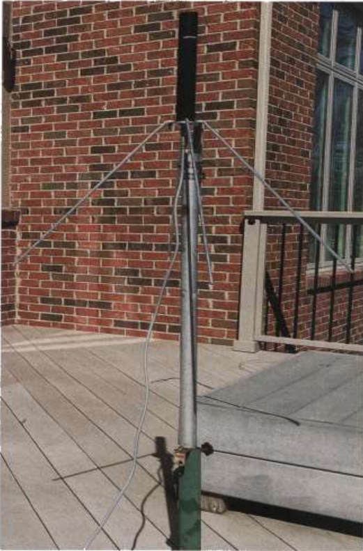
Figure 8 — The COMPACTenna 2M/440+ balcony station installation with CompacCounterpoise ground plane.
